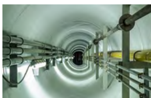
Low pressure pipelines
